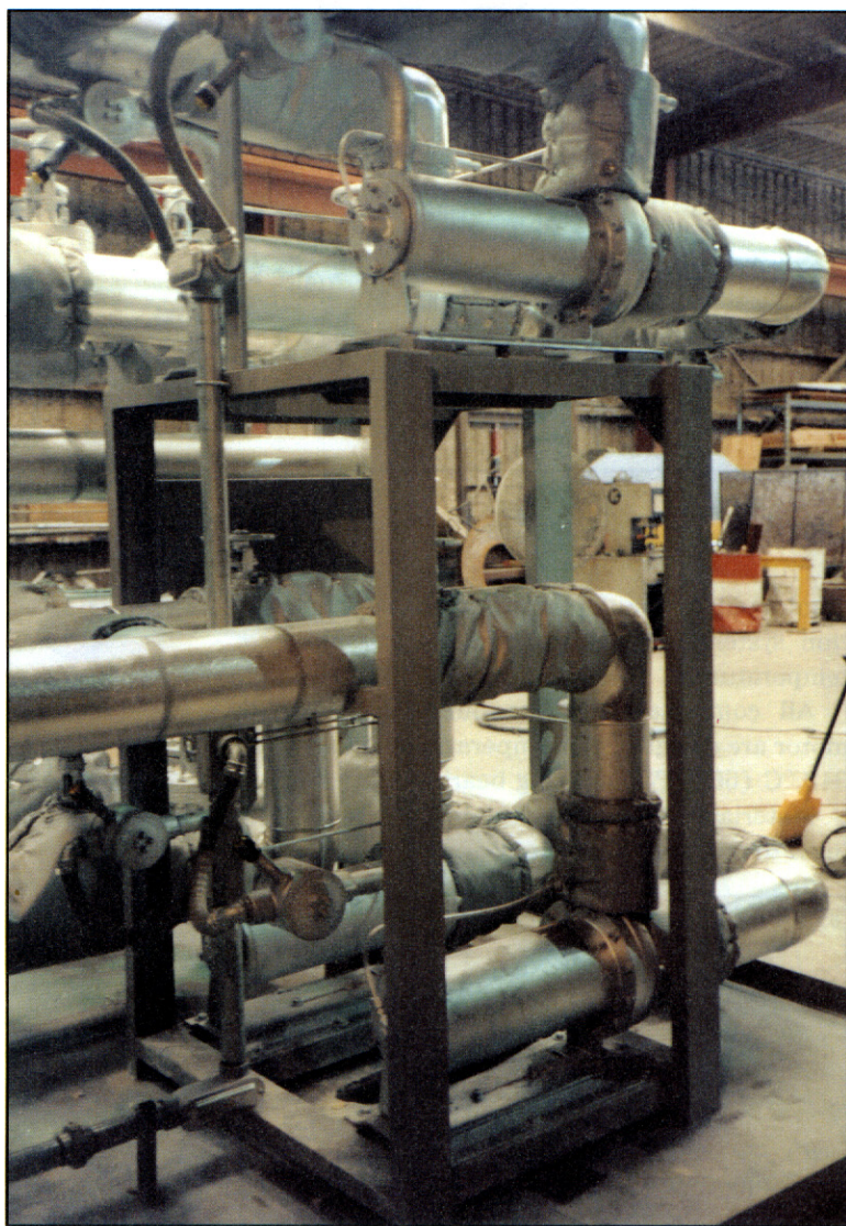
Four Crane Co., Chempump Division, canned motor pumps in a high temperature application. Photo courtesy of Texas Systems and Controls, Houston, TX, USA.
